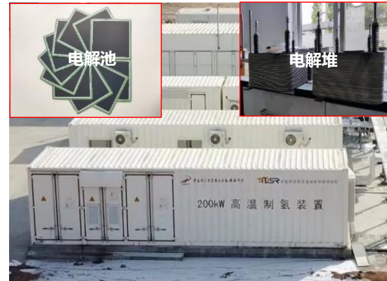
200kW-SOEC制氢系统 Hydrogen production system
